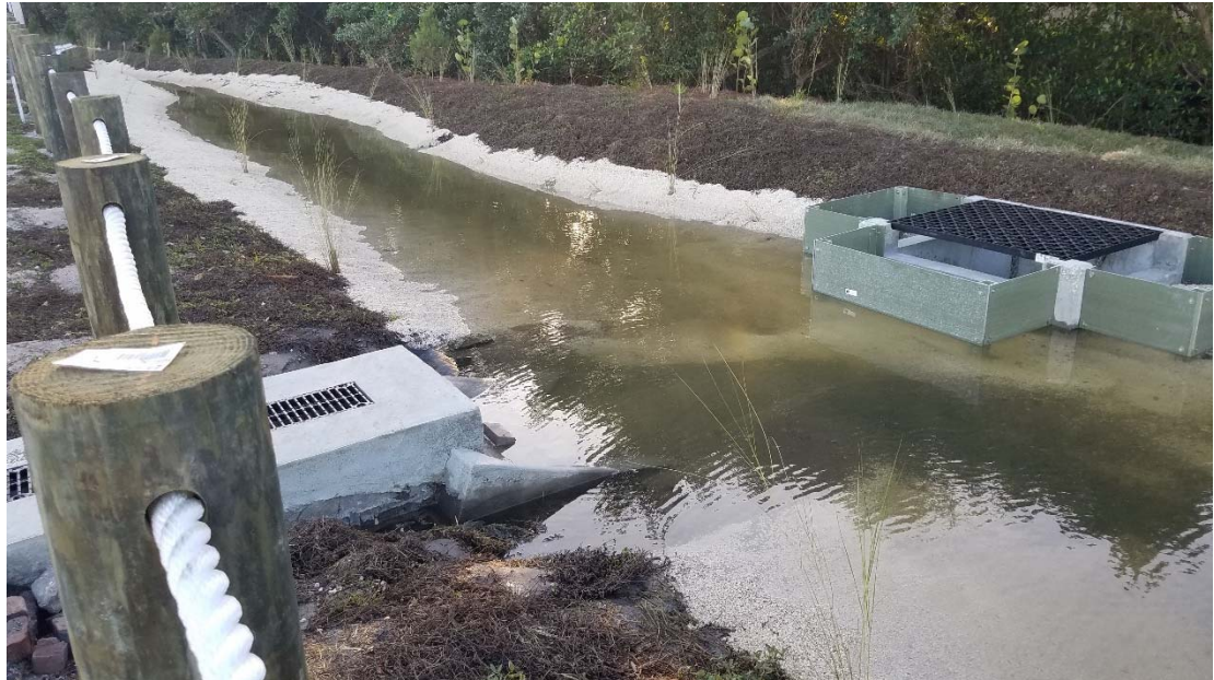
Bioswale – In Operation Parking Lot Flume and Control Box
