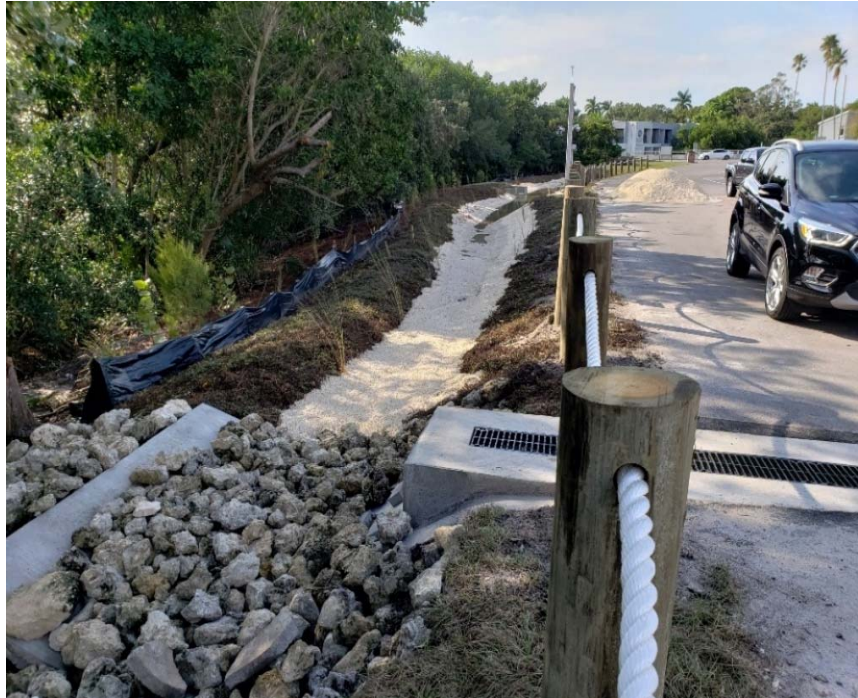
Bioswale Treatment Area and Parking Lot Trench Drainage Box
