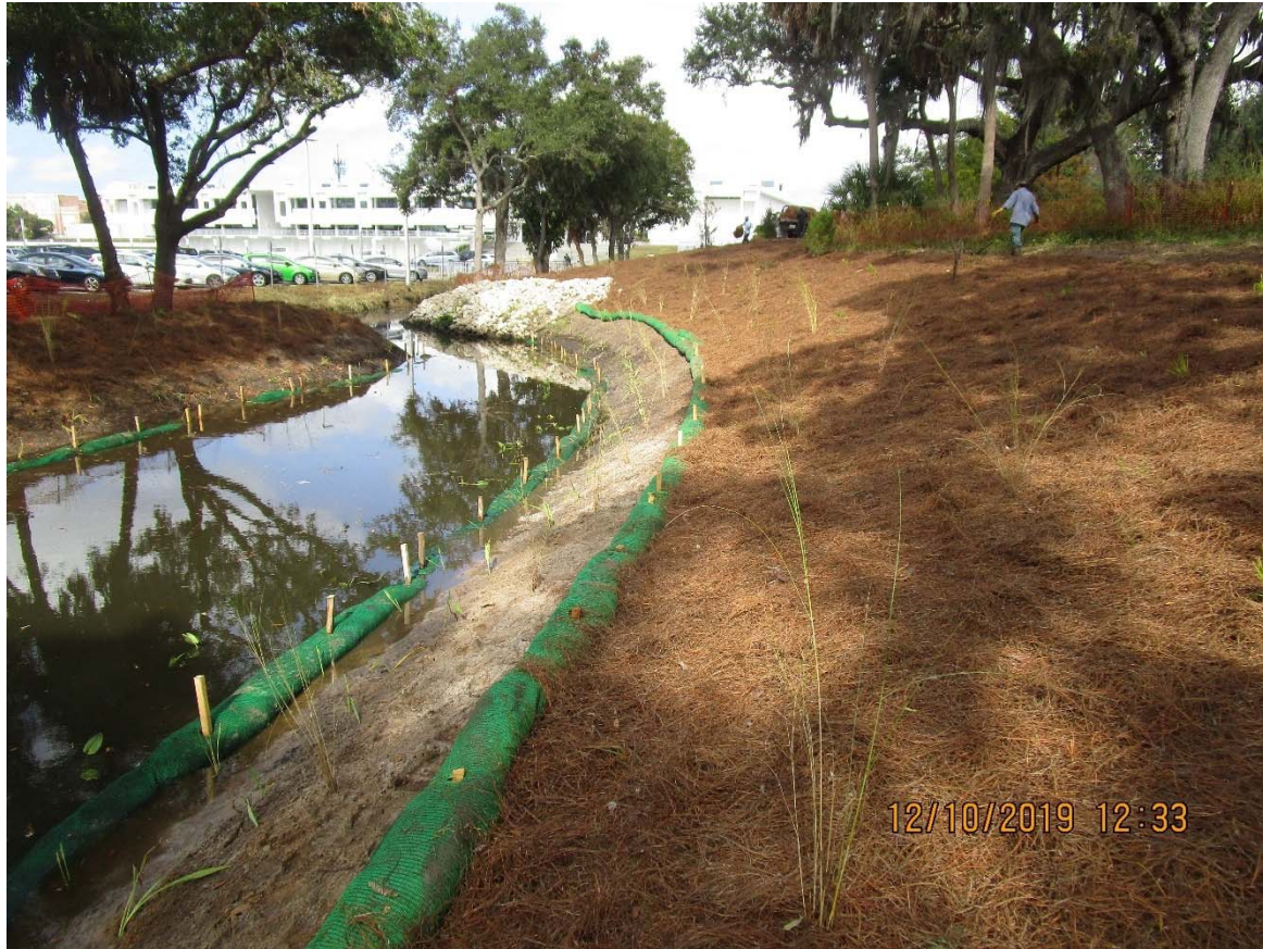
Offline Filter Marsh and Native Plantings
