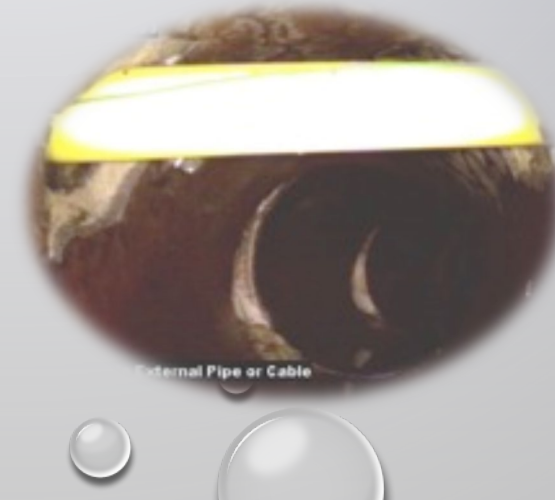
Cross-Bored Gas Line
